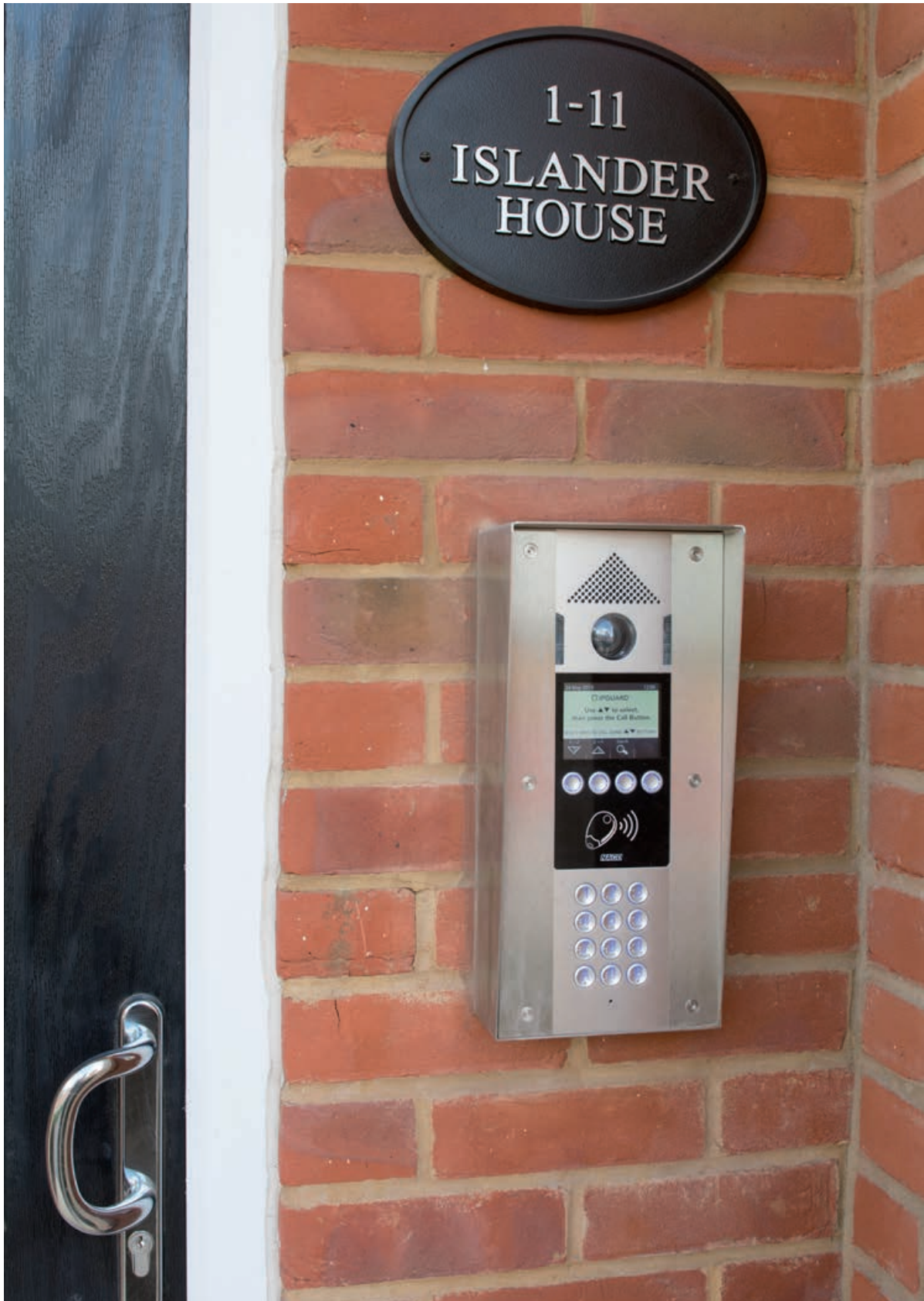
Main entrance secured using an IPGUARD® Smart Visitor panel. Residents answer calls from visitors on their own communications devices. It is so simple, they use the devices they want to use!
