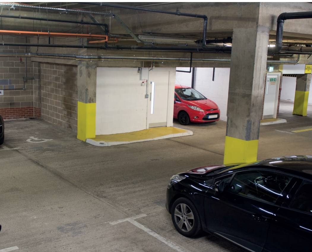
Doors from car park into the building are proximity reader controlled.
